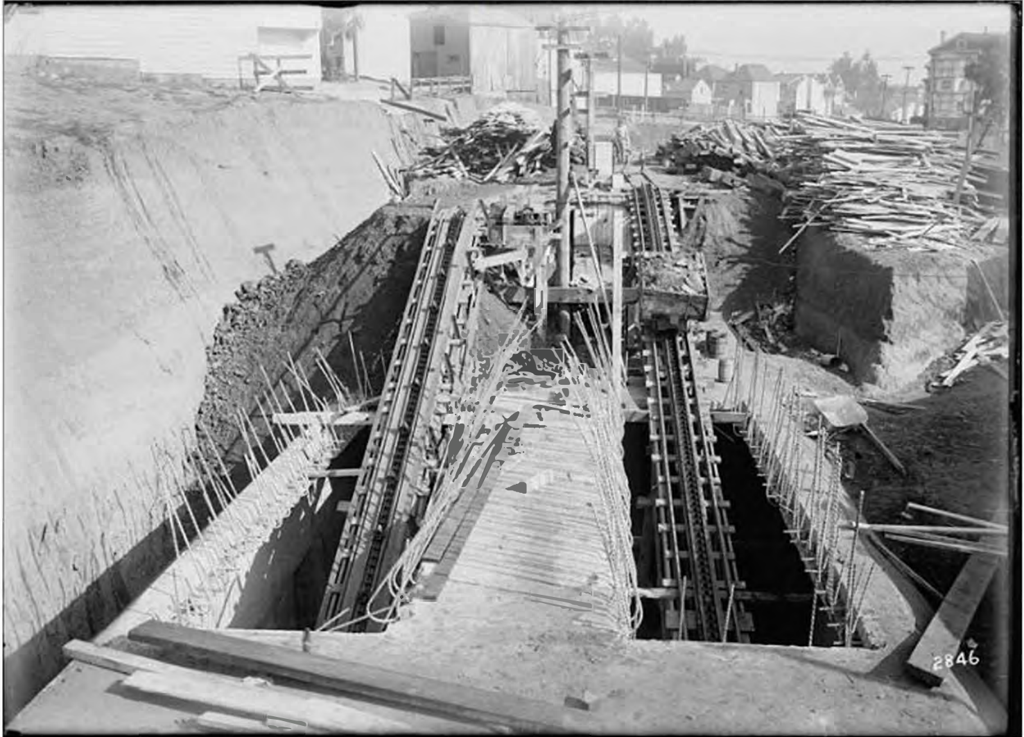
A small rail conveyor system was built to haul away excavated dirt on the eastern portion of the tunnel. This view looks east down Market Street near Diamond Street.
