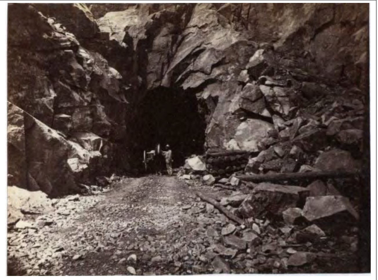
Hart 198. East Portal; of Summit Tunnel, Western Summit. Length 1,660 feet. The photo shows a Chinese worker with a horse cart removing spoils from the tunnel after a blast.
