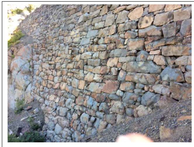
Detail of China Wall with hand laid stone without mortar. The track above operated from 1868 until 1993, carrying heavy modern trains without movement or damage to the wall.
