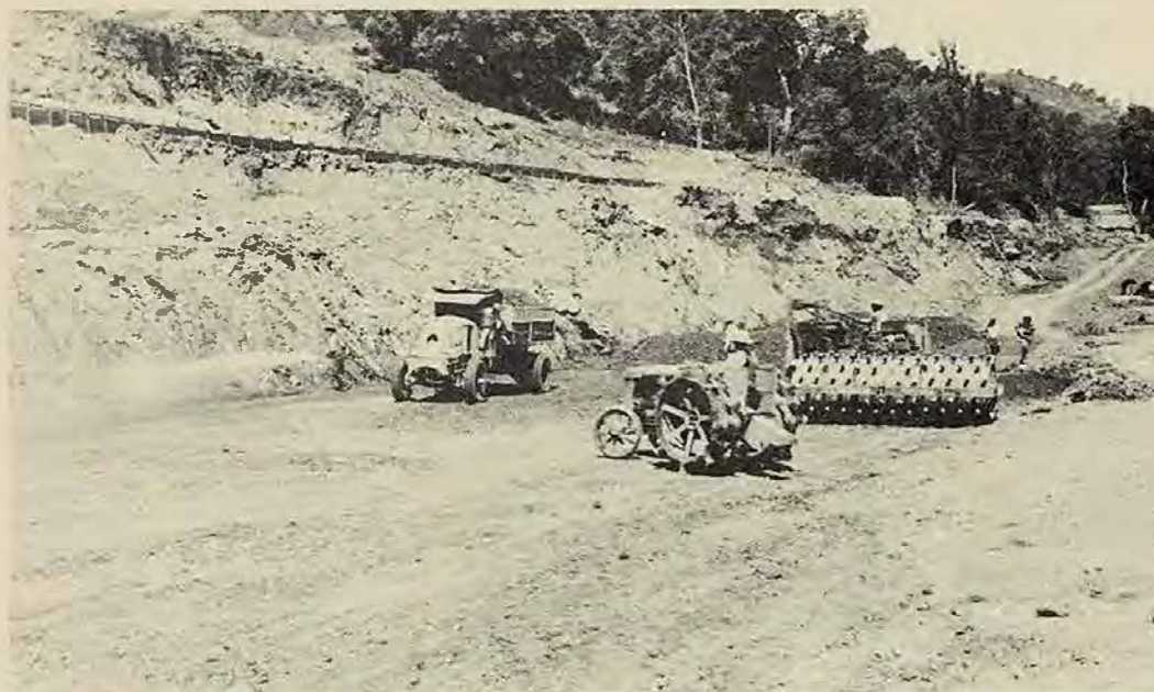
Construction of Coyote Dam and five others for the Water Conservation District provided much needed work for the Santa Clara Valley during the Great Depression.
