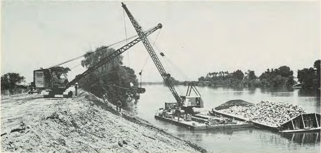
Levee repair, slope dressing and rip-rapping at Merrit Island on the Sacramento River.
