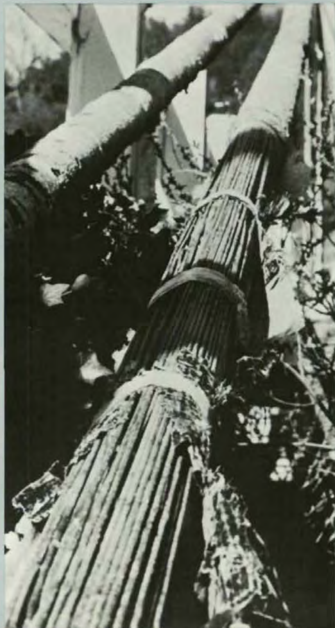
Cable covering deterioration near the anchorage. Exposed wires show little evidence of deterioration.
