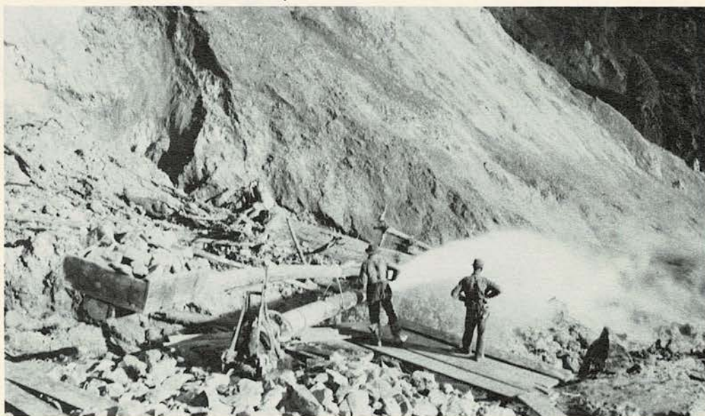
Application of an hydraulic monitor on the Oregon Mountain highway cut near Weaverville.
