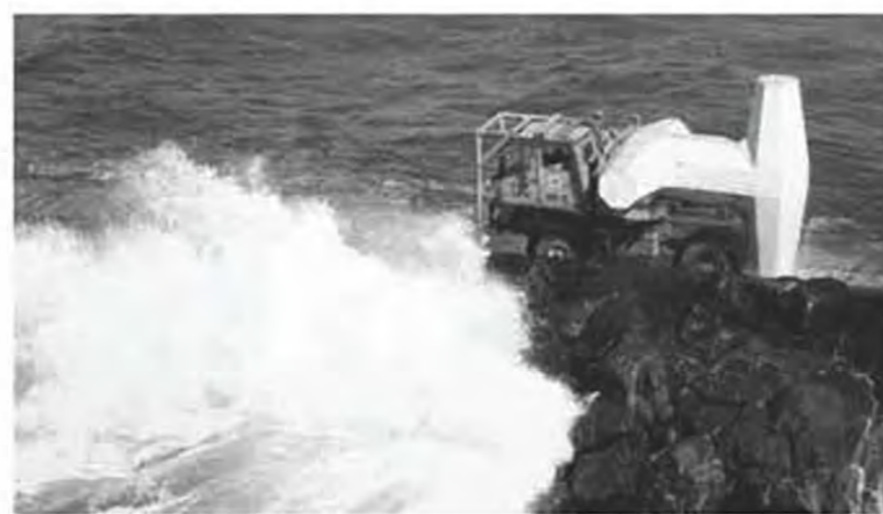
TOP IN THE EARLY 1960S, THE U.S. ARMY CORPS OF ENGINEERS PLACED 100-TON BLOCKS ON THE SOUTH JETTY. THEY WASHED AWAY WITHIN FIVE YEARS, ABOVE AN INTREPID CONTRACTOR HAULS A 42-TON DOLOS OUT TO THE HEAD OF THE SOUTH JETTY, CIRCA 1971. PHOTOS COURTESY OF THE U.S. ARMY CORPS OF ENGINEERS
