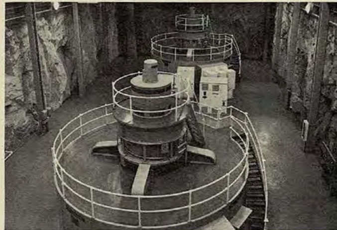
Located 500 feet below ground, the vast cavern of Haas Powerhouse contains machines capable of producing 144 megawatts of electricity.
