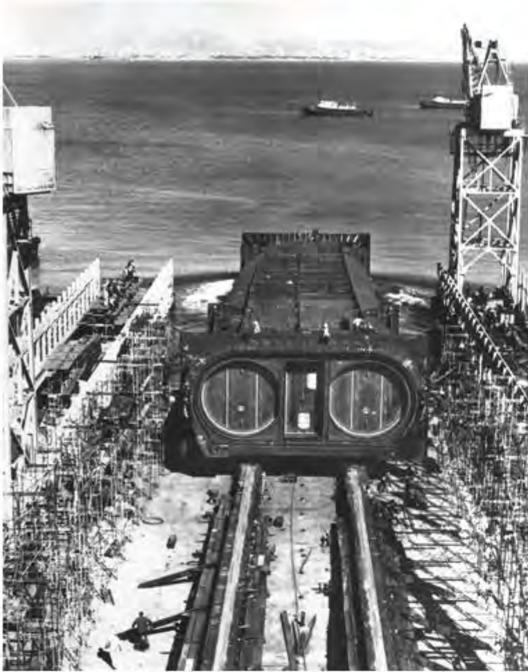
A section of the Transbay Tube being lowered into San Francisco Bay.
